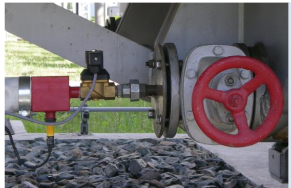
VIMAP RCID inlet line - Connection to power transformer's bottom valve
